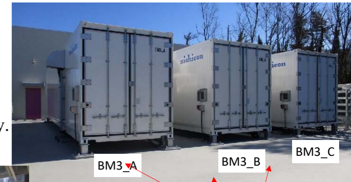
Capacitor Banks for BM3
